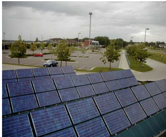
Minnesota Valley Transit Authority (10.0 kW) Burnsville, MN
